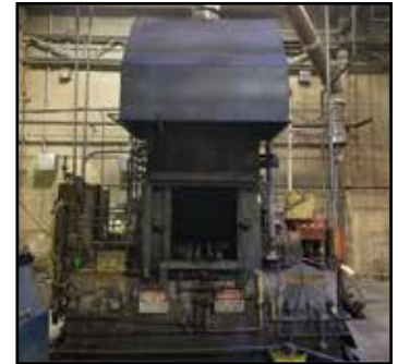
SURFACE COMBUSTION Allcase Super Proelectric Furnace
